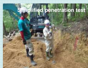
Simplified penetration test Development of the technology for opening sturdy and low-cost strip roads
